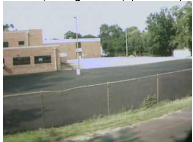
Before they left for the day at 4:20pm half to the base layer was in place
